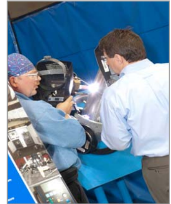
WWM affiliate PCI Energy Services provides field welding, custom tooling and machining services. Here, Welding Supervisor Peter Huckstep demonstrates an orbital welding system using Arc Products Power Supply during the WWM Open House.
